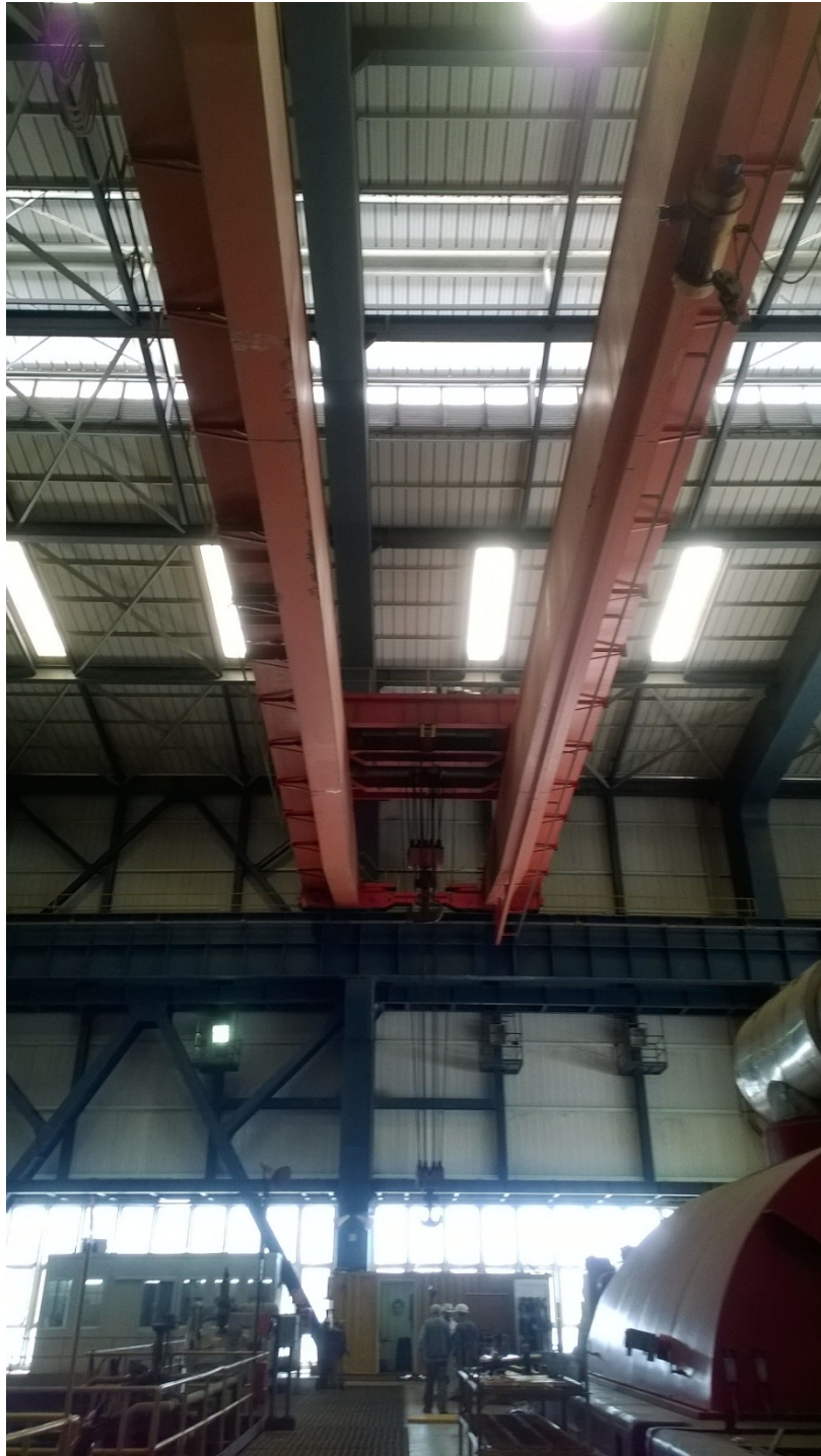
Figure 19. Trolley of the overhead crane (Edipower – a2a Group).
