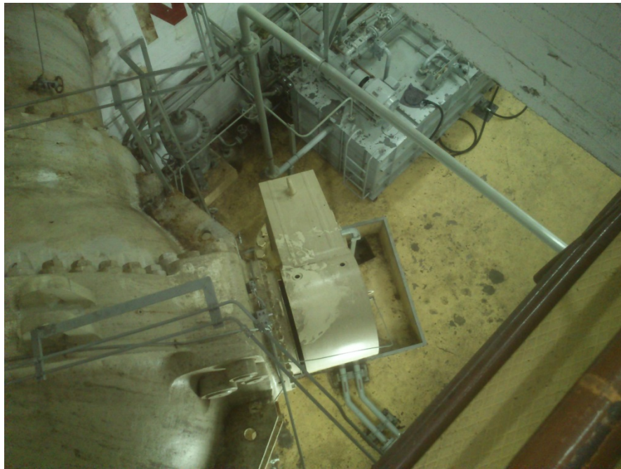
Figure 13. The lowest level of machine hall served by the selected crane (view from the crane cabin level).
