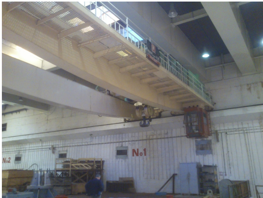
Figure 9. Machine hall and selected crane in HEPP "Bajina Basta".
