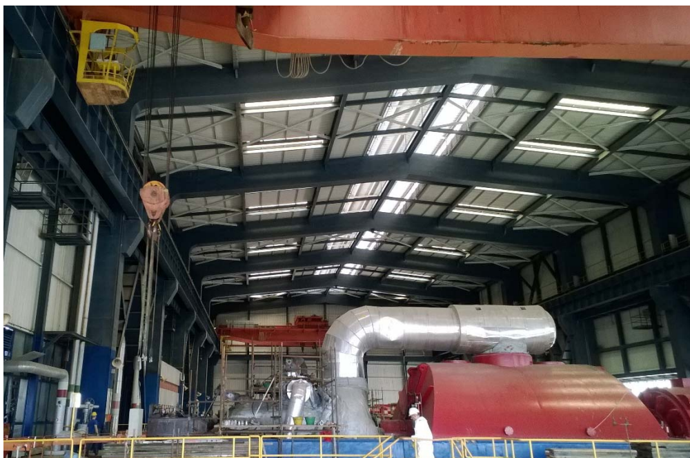
Figure 8. Machine hall and selected crane of the Edipower Company.
